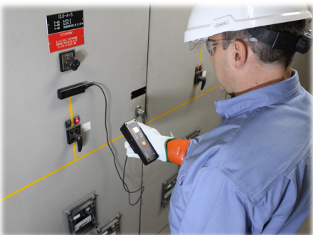
Contact acoustic sensor for partial discharge detection in metalclad cabinets
